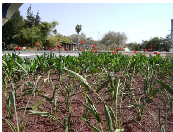
Figure 1. Wastewater Treatment System (field view).
